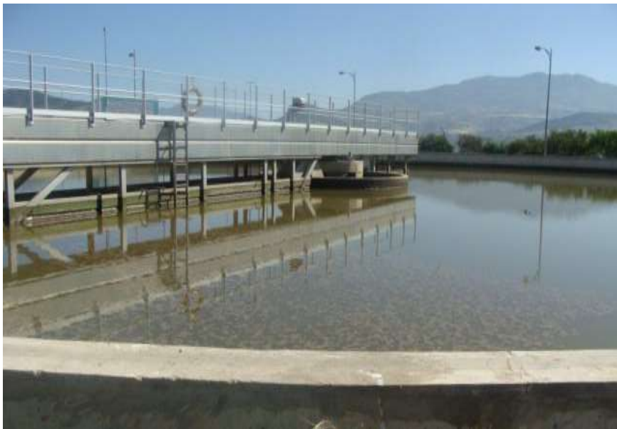
Figure 16: Clarificateur de la station de Sidi Merouane.
