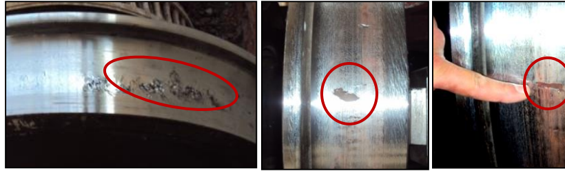
Figure1. The different defects on tread (Photos taken in the railway maintenance workshop (RMW) SMK Constantine .
