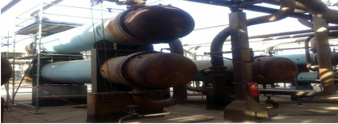
Fig. 1 Picture of the E101 CBA heat exchanger
