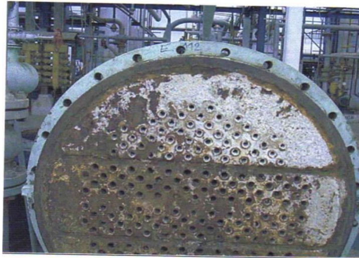
Fig 2 Example of a fouling exchanger
